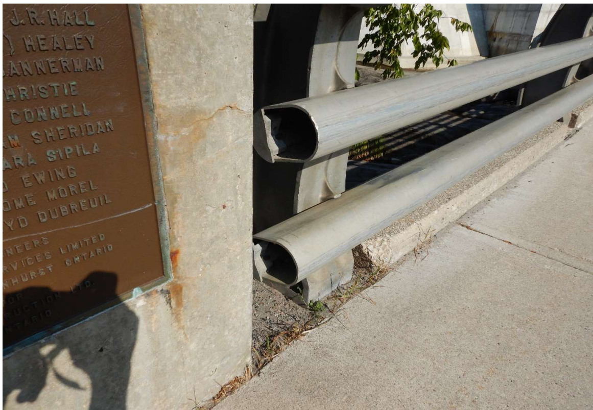
Description of Photo: East Rail, Note Missing End Caps
