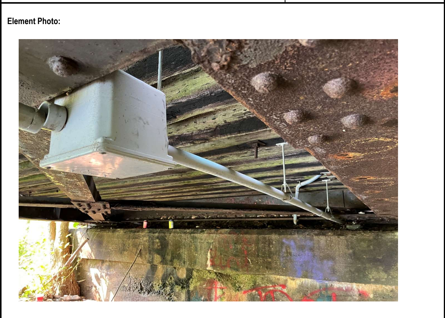
Description of Photo: Electrical utility
