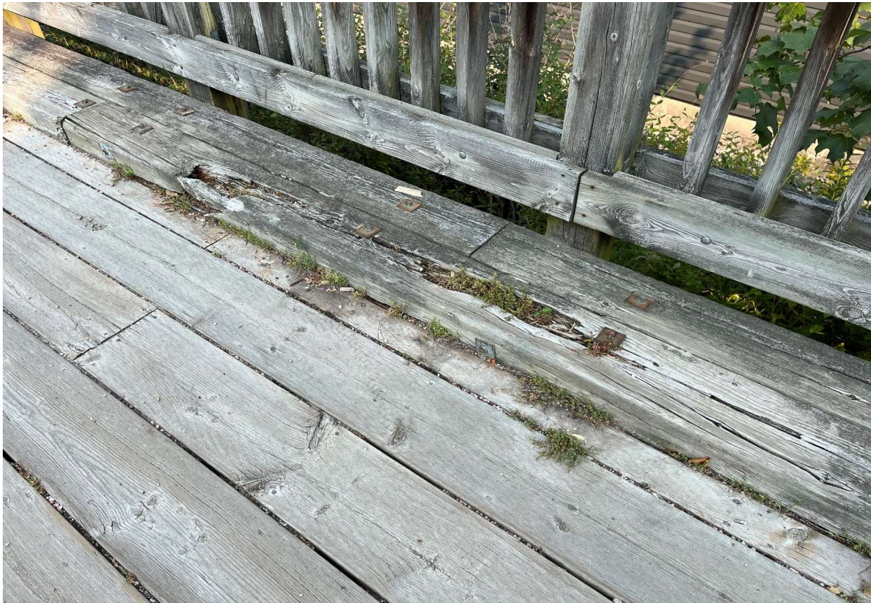
Description of Photo: Rotten curb
