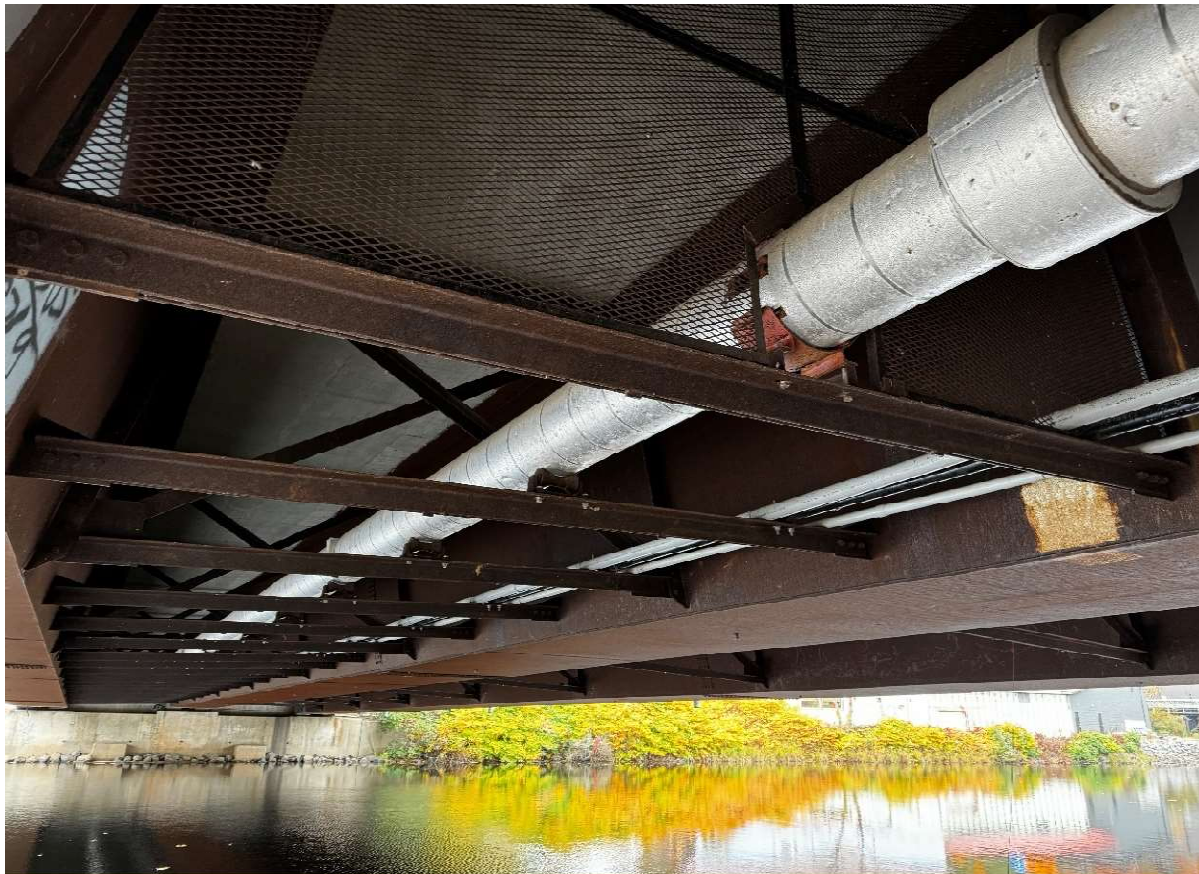
Description of Photo: Utilities
