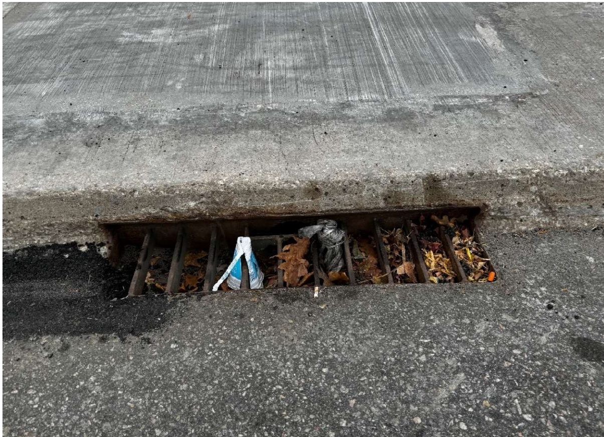
Description of Photo: Drainage
