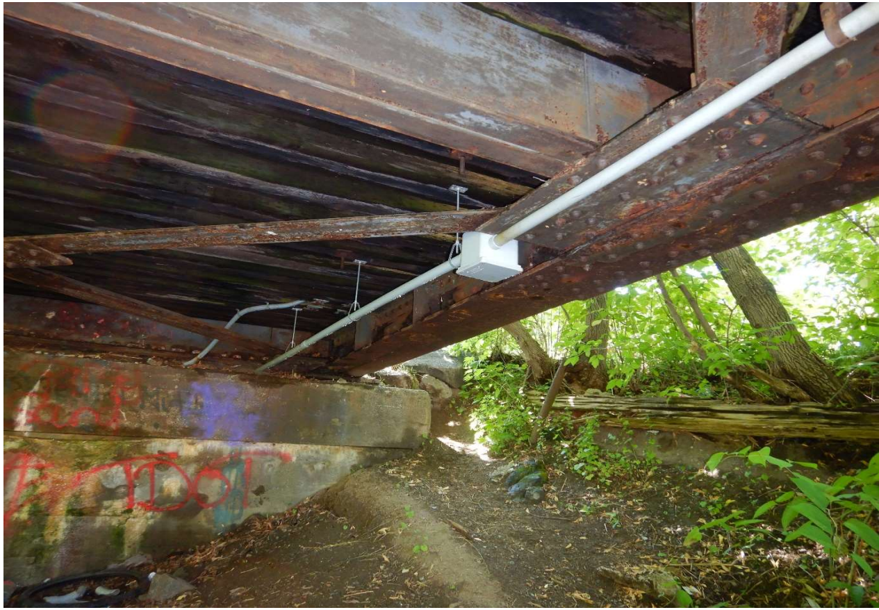
Description of Photo: Electrical Utilities
