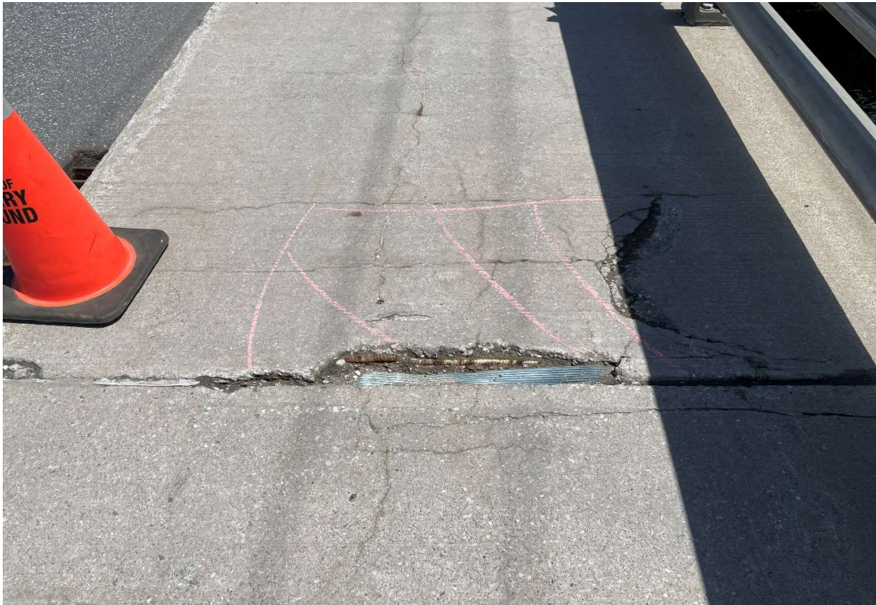
Description of Photo: Sidewalk Concrete Spall and Delamination
