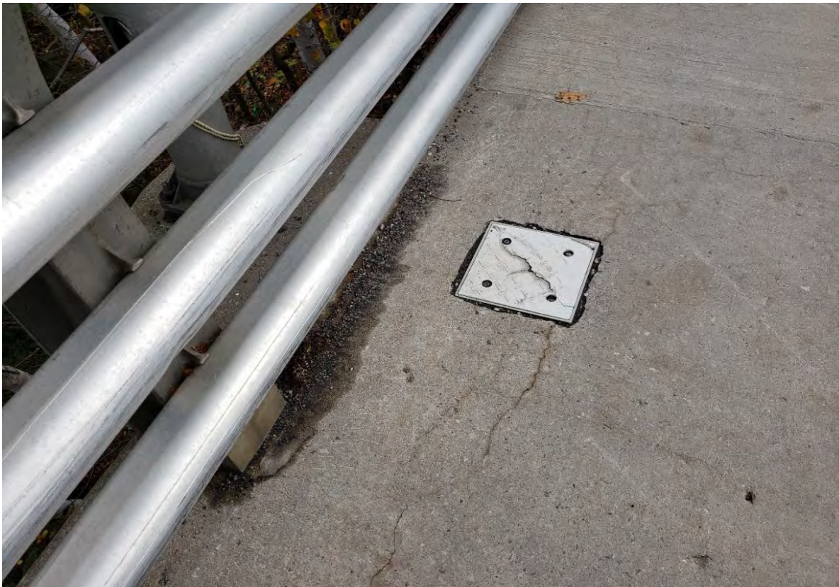
Description of Photo: Photo 27 - Utilities
