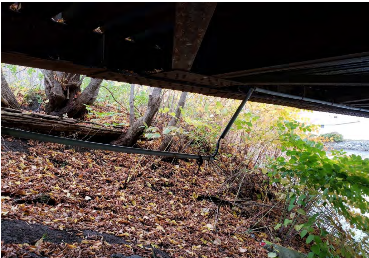
Description of Photo: Photo 17 - Utilities
