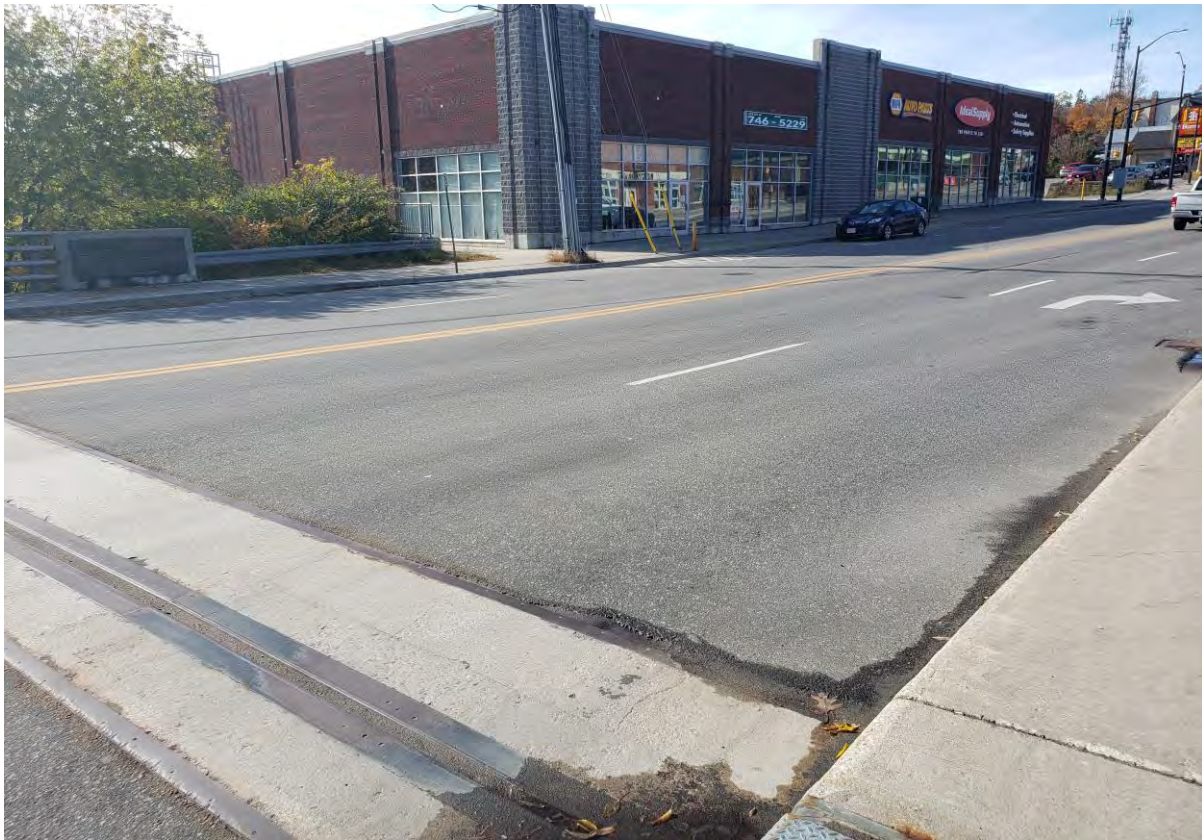
Description of Photo: Photo 3 - Approach Slab.jpg
