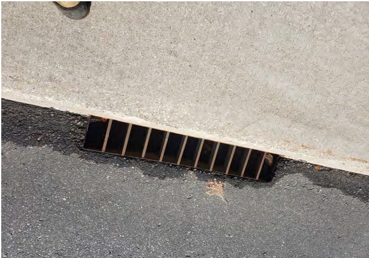
Description of Photo: Photo 16 - Drains.jpg
