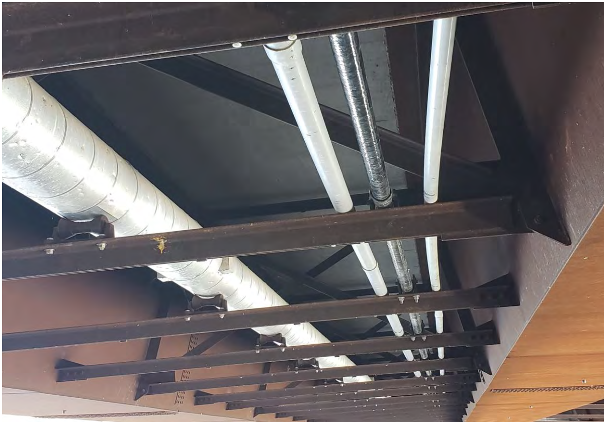
Description of Photo: Photo 28 - Utilities.jpg
