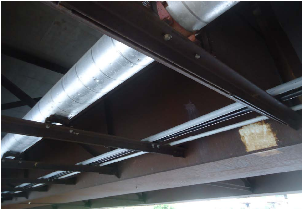
Description of Photo: Photo 81 - Utilities
