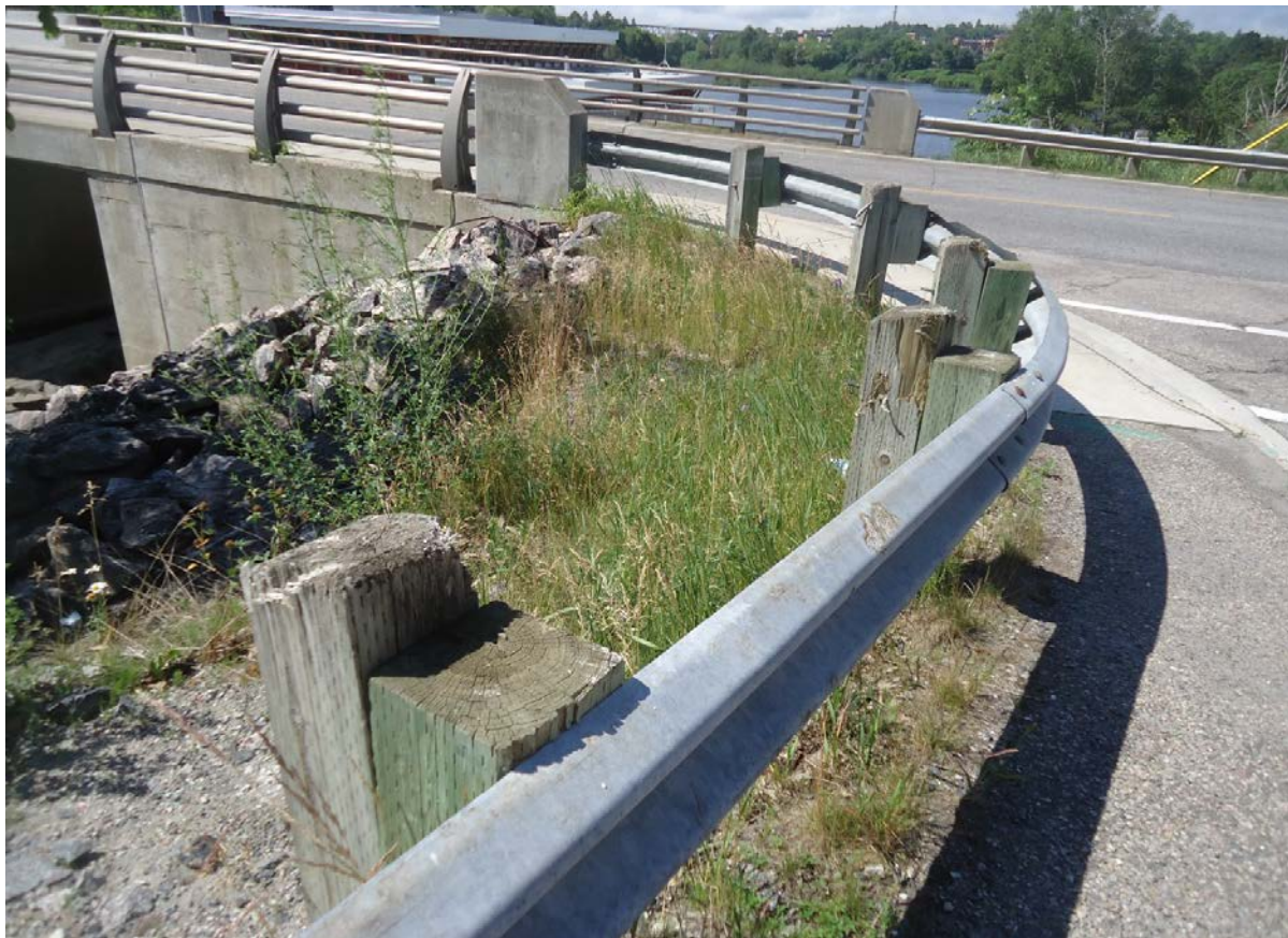
Description of Photo: Photo 37 - Northeast Approach Barrier
