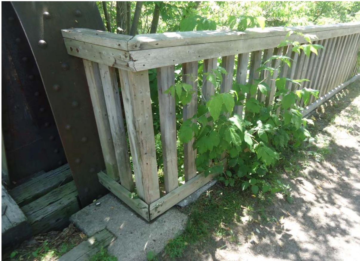
Description of Photo: Photo 34 - Southwest Approach Barrier
