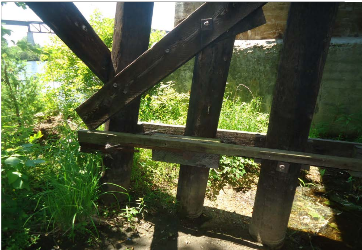
Description of Photo: Photo 44 - Timber Bracing
