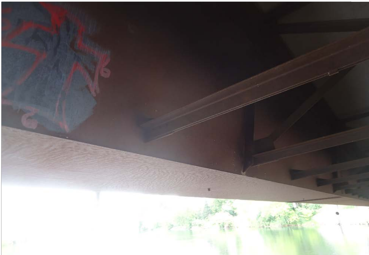
Description of Photo: Photo 29 - Cross Bracing
