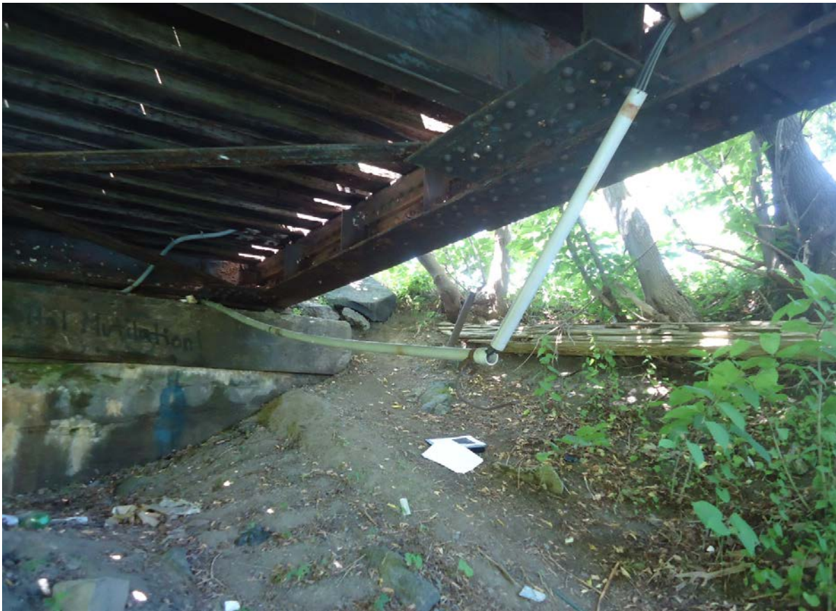
Description of Photo: Photo 33 - Broken Conduit
