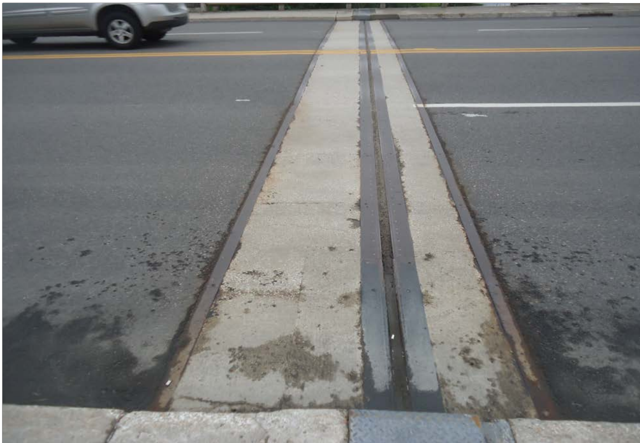
Description of Photo: Photo 20 - Steel Angle Armouring
