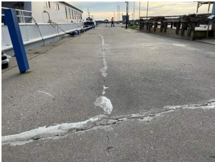
27- Structure C – Settled Area, Stn 0+085 to 0+117.8
