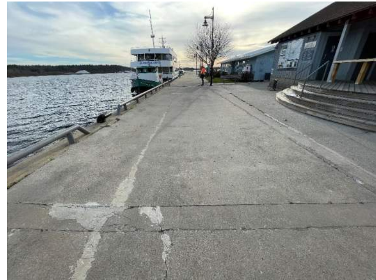
14- Structure C – Longitudinal Crack extending past Settlement
