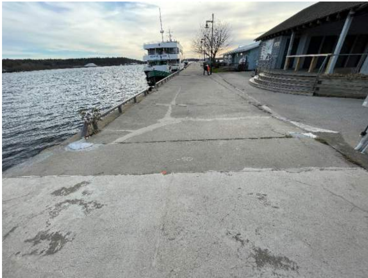
13- Structure C – Settled Area, Stn 0+048.3 to 0+069
