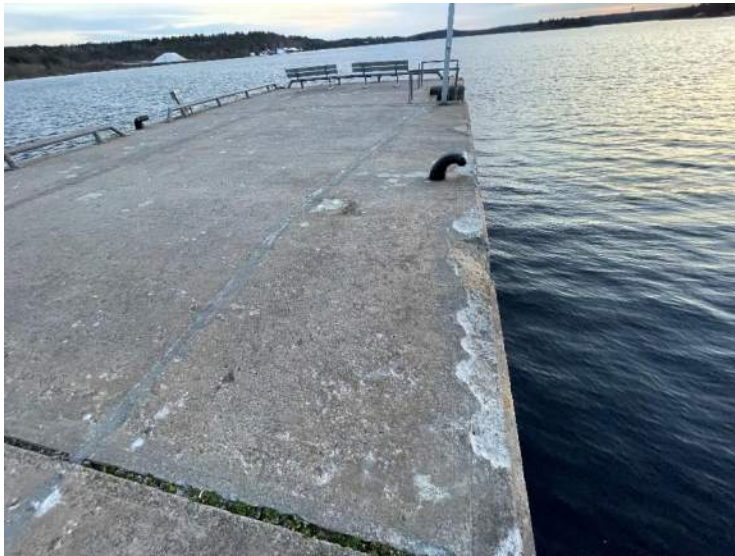
133- Structure D – Severe Scaling at West Edge, Stn 0+262
