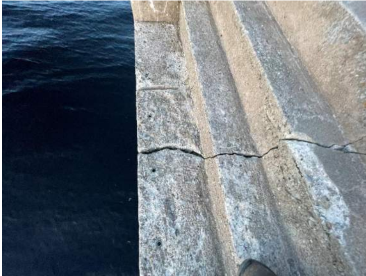
141- Structure D – Wide Crack at West Steps, Stn 0+270
