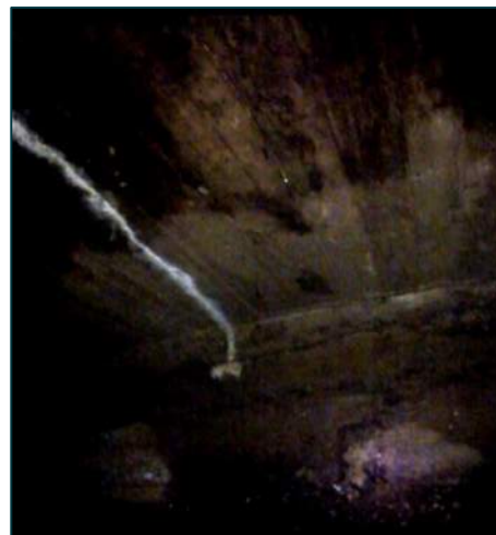
Location: STA 0+248.2 Transverse Distance to Nearest Edge: 2.31 m to East Concrete Deck Thickness: ± 508 mm Fill Level to Top of Concrete: ± 2.2 m Observations: Efflorescence, underside of medium crack at 0+251.
