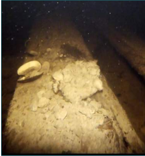
Location: STA 0+258.5 Transverse Distance to Nearest Edge: 2.71 m to West Concrete Deck Thickness: ± 508 mm Fill Level to Top of Concrete: ± 2.4 m Observations: Top of Pile Cap.
