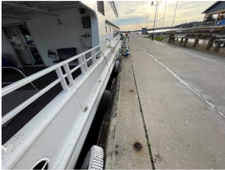
25- Structure C – Removed Curb Railing, Stn 0+087 to 0+093
