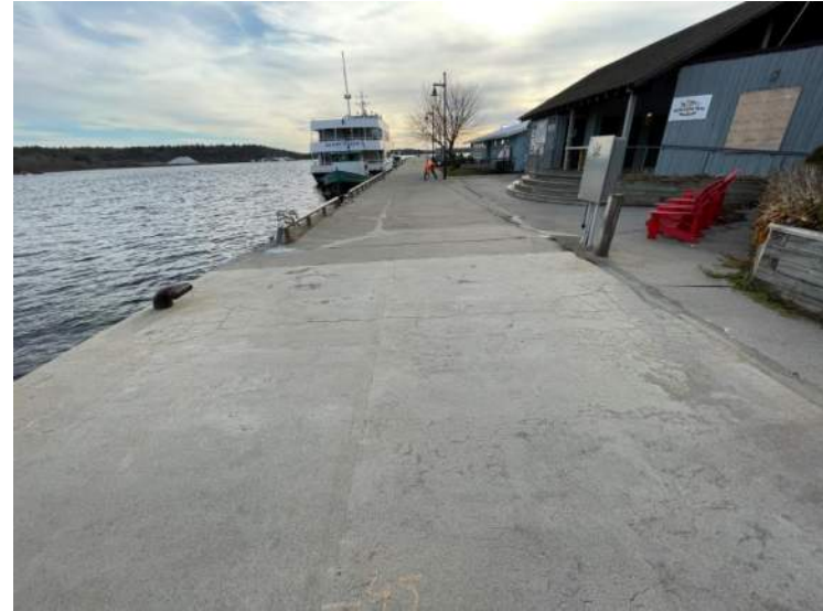
10- Structure B – Map Cracking at Concrete Deck, Stn 0+045
