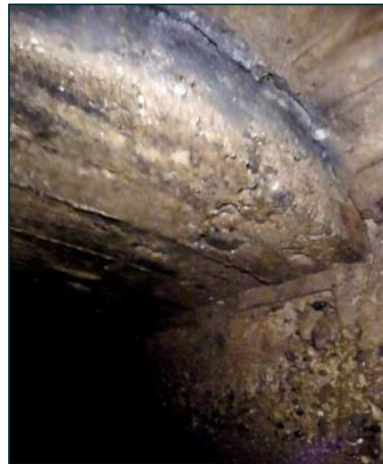
Location: STA 0+198.6 Transverse Distance to Nearest Edge: 1.59 m to West Concrete Deck Thickness: ± 508 mm Fill Level to Top of Concrete: ± 2.2 m Observations: Underside of south corner of buried slipway at 0+200.
