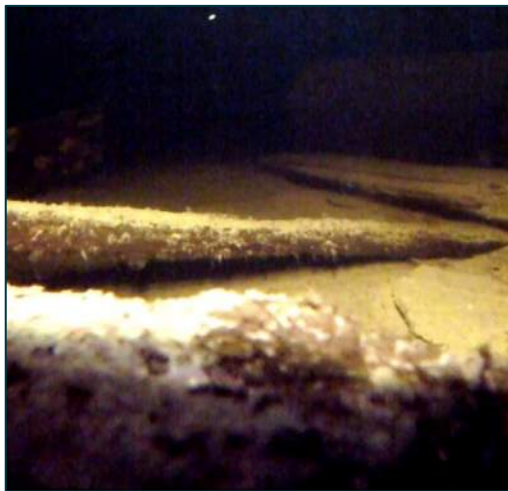
Location: STA 0+228.6 Transverse Distance to Nearest Edge: 3.04 m to West Concrete Deck Thickness: ± 508 mm Fill Level to Top of Concrete: ± 2.2 m Observations: Unidentified timber debris above fill.
