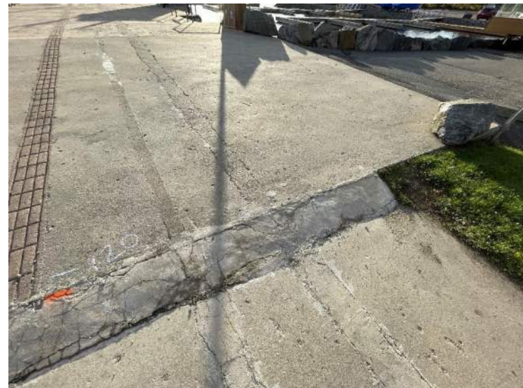
36- Structure C – Delamination at Transition to Structure D
