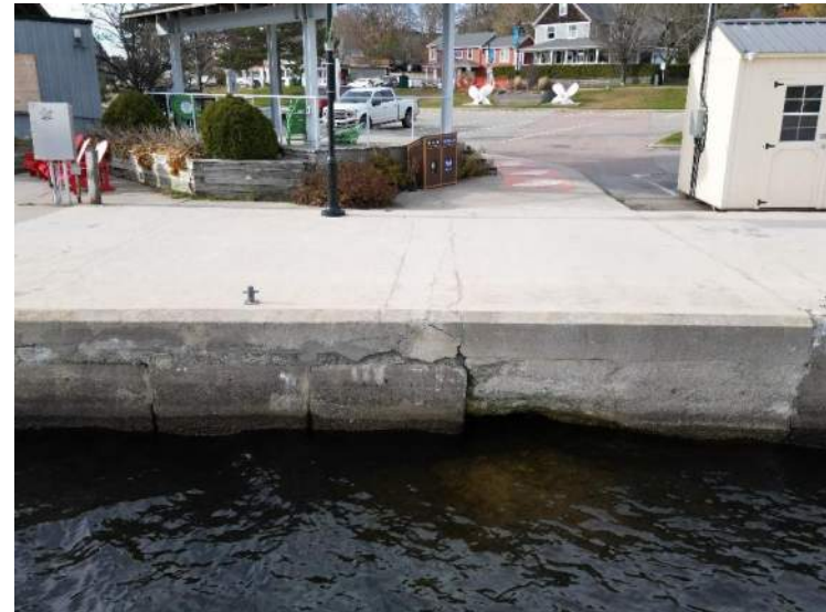
144- Structure B – Fill Washout from Deteriorated Wall, Stn 0+039.5
