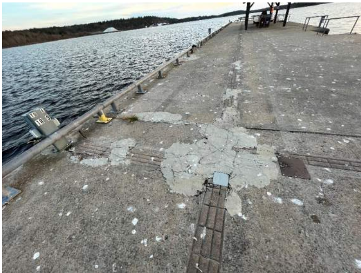
115- Structure D – Delaminated Patchwork, Stn 0+228
