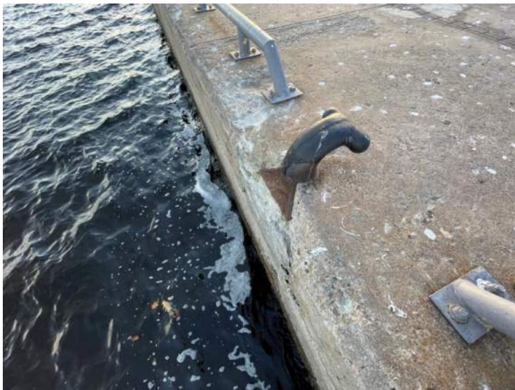
91- Structure D – East Bollard condition, Stn 0+190
