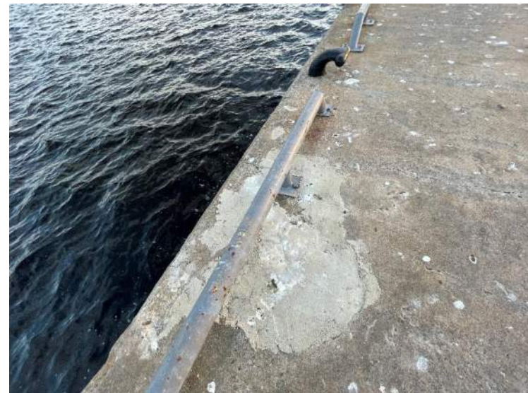
120- Structure D – East Bollard and Delamination, Stn 0+236
