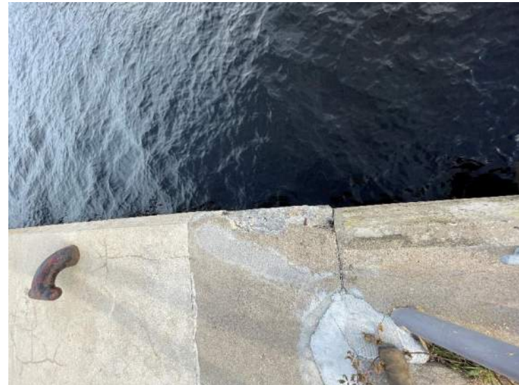
12- Structure B – Spall and Patch at Transition, Stn 0+048.3
