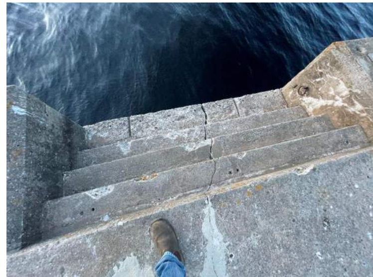
140- Structure D – Wide Crack at West Steps, Stn 0+270
