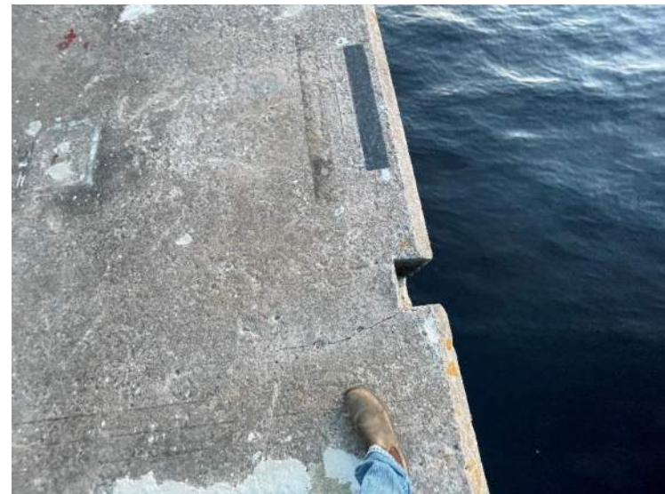
128- Structure D – Knockout in Concrete Deck (West), Stn 0+249
