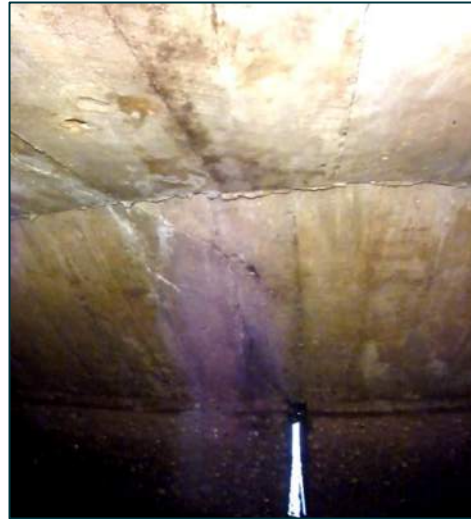
Location: STA 0+261.7 Transverse Distance to Nearest Edge: 2.31 m to West Concrete Deck Thickness: ± 508 mm Fill Level to Top of Concrete: ± 2.4 m Observations: Very wide crack at 0+271 noted in above water inspection. Visibility here indicates crack penetrates all the way through the concrete deck
