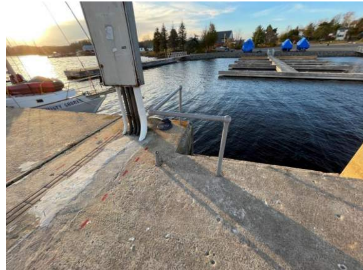
86- Structure D – Missing Railing Post at West Steps, Stn 0+180
