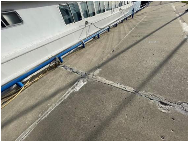
31- Structure C – Delamination over Buried Conduit, Stn 0+097
