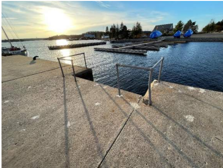
71- Structure D – Bent Railing at West Steps, Stn 0+161 to 0+164
