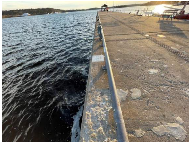
87- Structure D – Severe Scaling at East Edge, Stn 0+176
