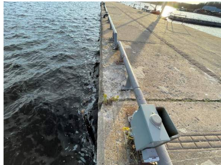
76- Structure D – Severe Scaling at East Edge, Stn 0+168
