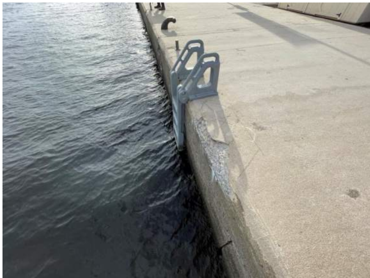
7- Structure B – Plastic Ladder and Delamination, Stn 0+32
