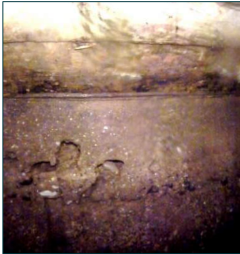
Location: STA 0+129.7 Transverse Distance to Nearest Edge: 1.65 m to East Concrete Deck Thickness: ± 508 mm Fill Level to Top of Concrete: ± 1.5 m Observations: Severe void due to deteriorating concrete on parapet.
