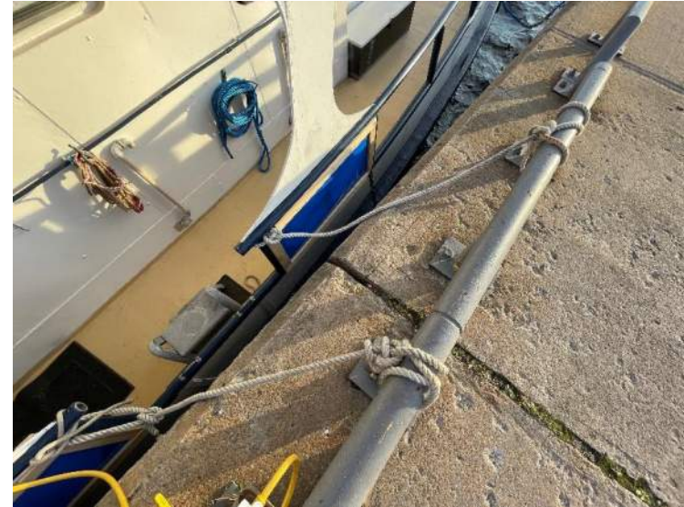
66- Structure D – Vegetation Growth in Expansion Joint, Stn 0+151
