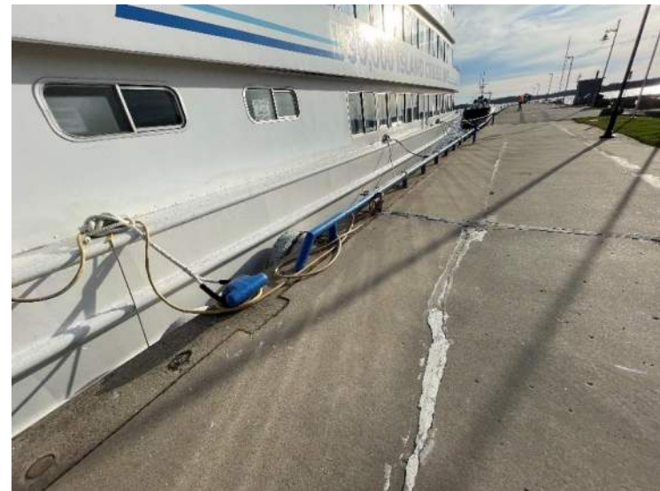
28- Structure C – Settled Area, Stn 0+095
