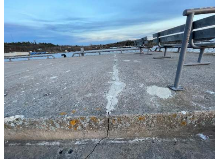
142- Structure D – Crack at West Steps extending East, Stn 0+270
