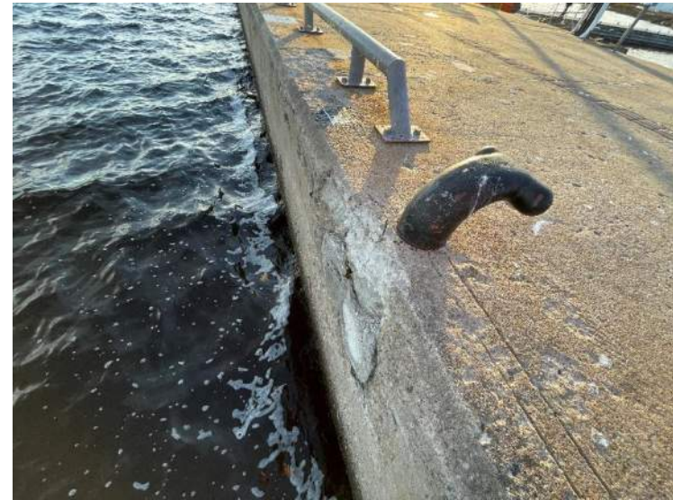
82- Structure D – East Bollard condition, Stn 0+175
