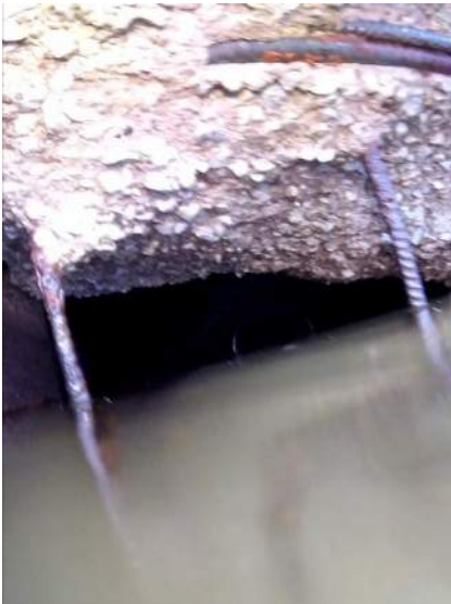
145- Structure B – Closeup of Wall Opening, Exposed Rebar, Stn 0+039.5
