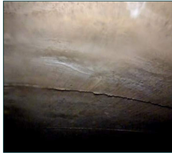
Location: STA 0+263.4 Transverse Distance to Nearest Edge: 2.44 m to West Concrete Deck Thickness: ± 508 mm Fill Level to Top of Concrete: ± 2.2 m Observations: Underside of deck, typical.
