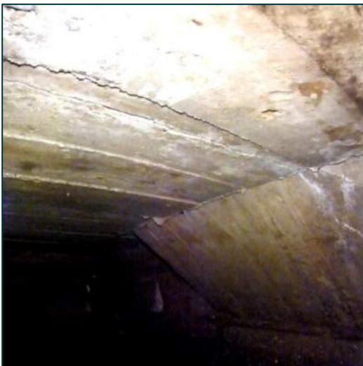
Location: STA 0+261.7 Transverse Distance to Nearest Edge: 2.31 m to West Concrete Deck Thickness: ± 508 mm Fill Level to Top of Concrete: ± 2.4 m Observations: Very wide crack at 0+271 noted in above water inspection. Also visible is the transition in haunch dimensions from stairs to copewall.
