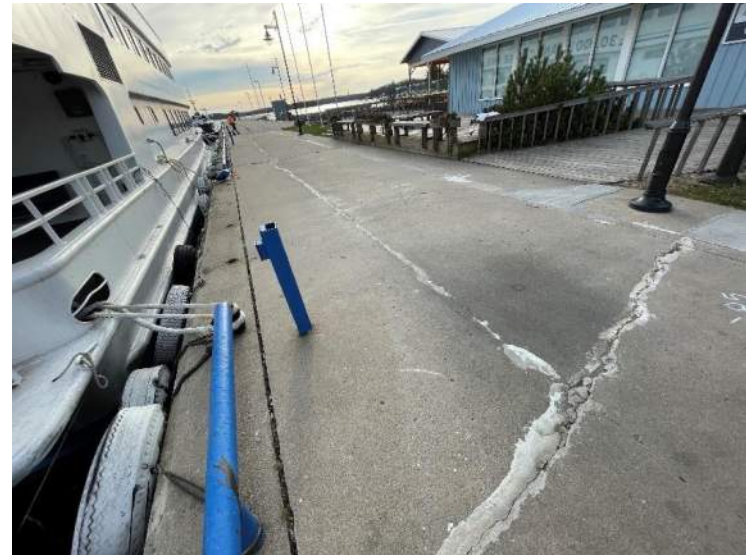
26- Structure C – Settled Area, Stn 0+085 to 0+117.8
