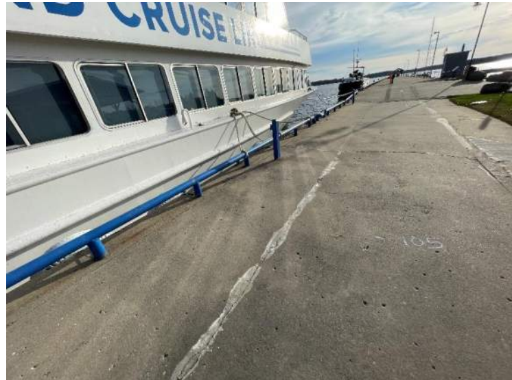
32- Structure C – Longitudinal Crack from Settlement, Stn 0+105
