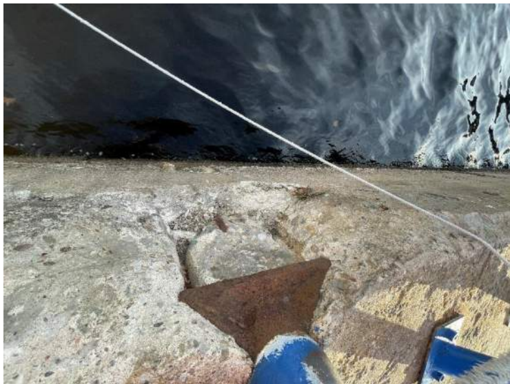
43- Structure D – East Face Bollard condition, Stn 0+129
